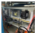
Electric control box 电控箱
